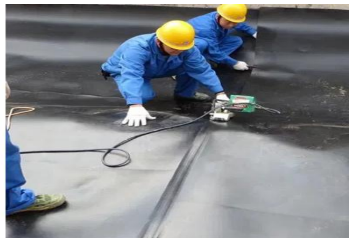
[Sewage Treatment Plant in Thailand]
