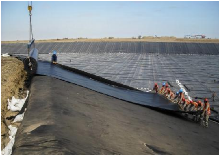
[Wastewater Treatment Plant in Algeria]
